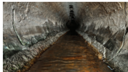
Figure 3. Sulfuric acid attacking the carbonates in cured concrete piping will compromise their capabilities as binding agents, turn solid pipe walls to flakey gypsum, and corrode the embedded reinforcing steel.
